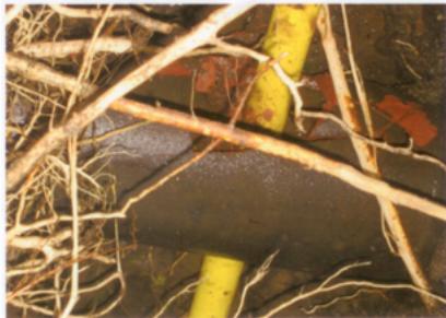
Fig. 1: Cross bore of sewer lateral with gas main
