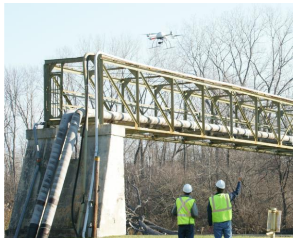
Figure 1: Close-up sUAS inspection of a pipeline crossing, difficult for routine inspection methods.
