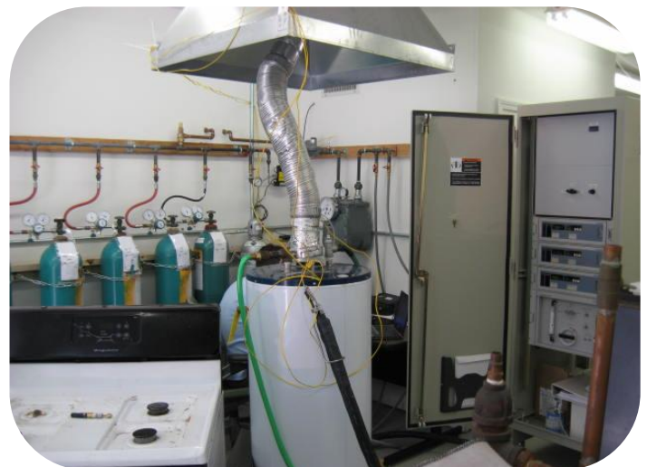
Residential appliance RNG testing with flame lifting identified (above) Siloxane compounds found in RNG (left)
