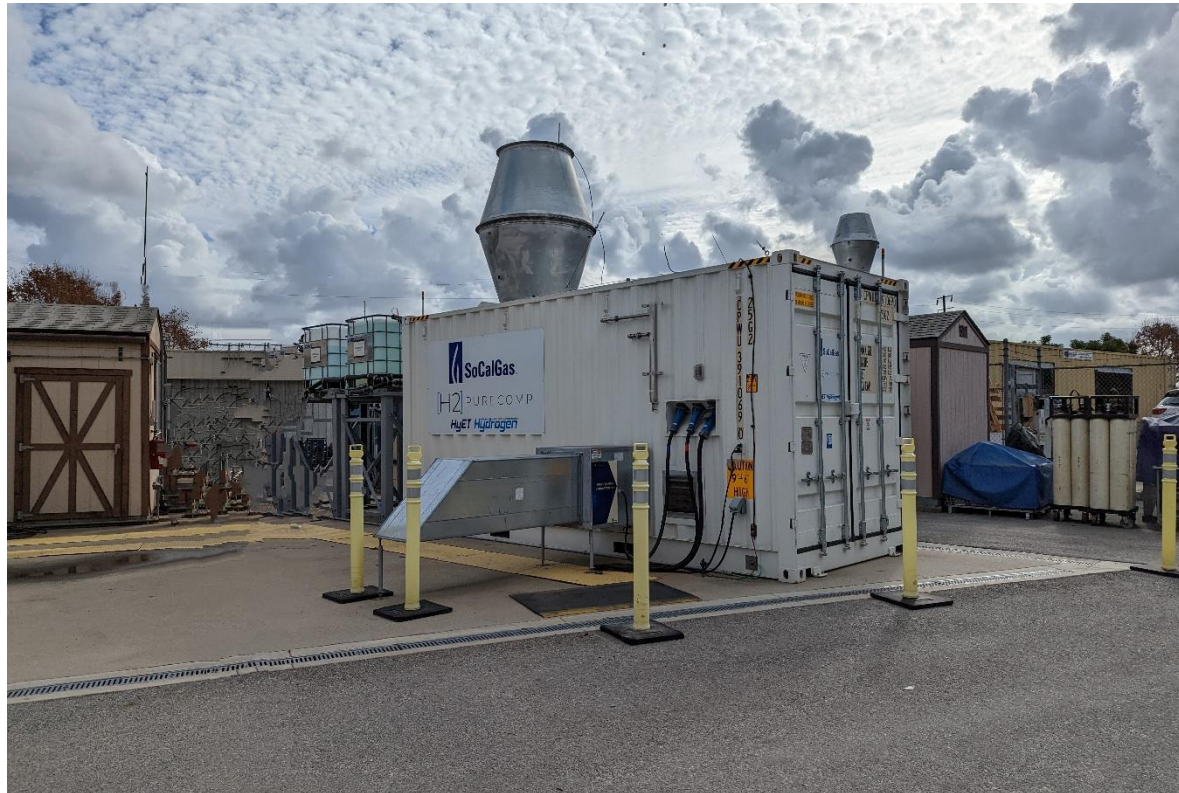
SoCalGas showcased a hydrogen - natural gas separation demonstration, H2 PureComp, at the NYSEARCH Quarterly December meeting in Pico Rivera, CA. SoCal's collaboration with HyET demonstrates state-of-the-art hydrogen separation technologies and how they are adapted to commercial end users.
