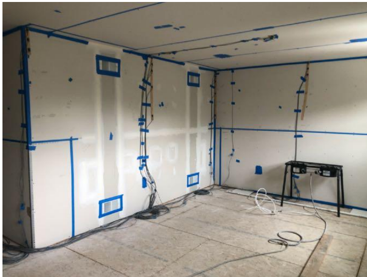
Figure 2: Installation of HVAC vents within structure; covered for no flow ventilation configuration.
